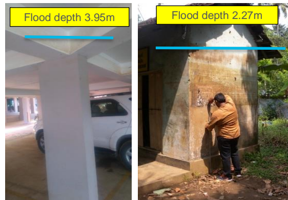
Figure 3. High water marks on residential buildings flooded from Periyar river waters
