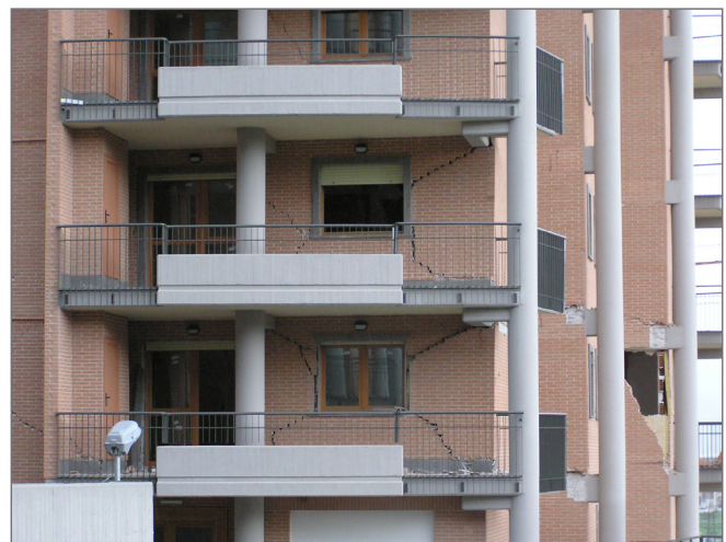
This modern building experienced cracking to brick infill walls but sustained no permanent damage to its reinforced concrete frame during the 2009 L'Aquila earthquake. (Source: AIR)
