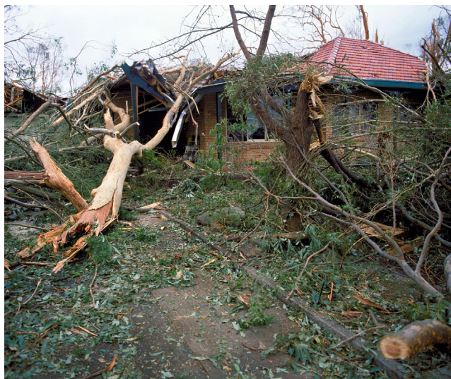
Top: Blue tarps cover half the roofs pictured due to damage from the 1999 Sydney hailstorm (Source: Commonwealth of Australia (Geoscience Australia) 2015). Bottom: This property suffered severe damage from straight-line wind.
